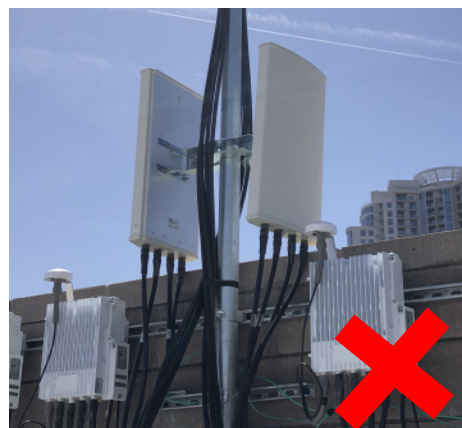
The GPS antenna is mounted on the front of the RF antenna
