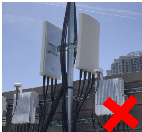
The GPS antenna is mounted on the front of the RF antenna
